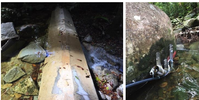
Weir and Sonde equipment installed in the creek at the DRO.
